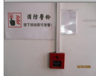
Photo of fire safety equipment Fire alarm button.JPG
