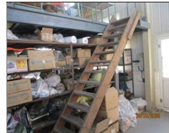
Photo of non-conformity NC7.11 The ladder did not equip with handrail.JPG
