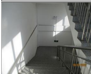
Photo of fire safety equipment Evacuation stair.JPG
