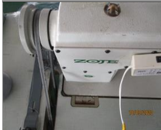
Photo of non-conformity NC7.17 Sewing machines were not equipped with belt guard.JPG
