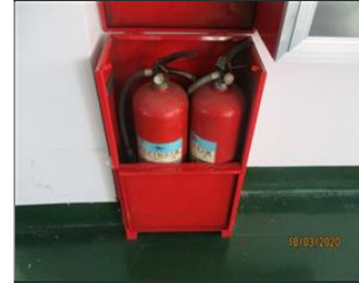
Photo of fire safety equipment Fire extinguishers.JPG
