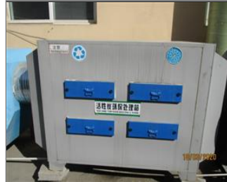
Photo of the inside of the main production hall Waste air treatment facility.JPG
