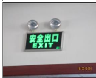
Photo of fire safety equipment Exit sign and emergency light.JPG
