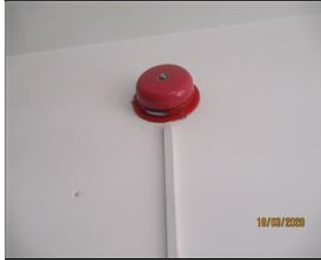
Photo of fire safety equipment Fire alarm.JPG
