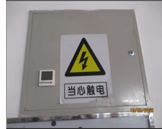
Photo of the inside of the main production hall Electrical cover.JPG
