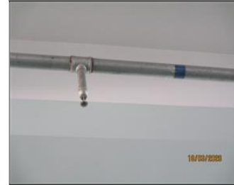
Photo of fire safety equipment Sprinkler system.JPG
