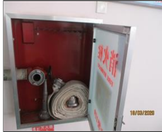
Photo of fire safety equipment Fire hydrant.JPG
